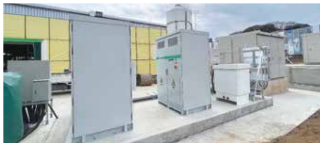
Renon DC ECube 157 kWh
