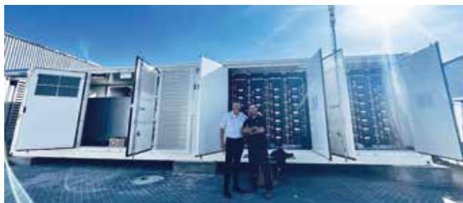
Renon Estation 744 kWh
