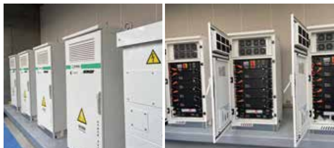
Renon DC ECube 38 kWh
