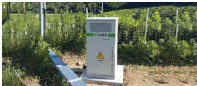
Renon DC ECube 38 kWh
