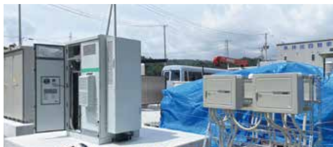
Renon DC ECube 157 kWh
